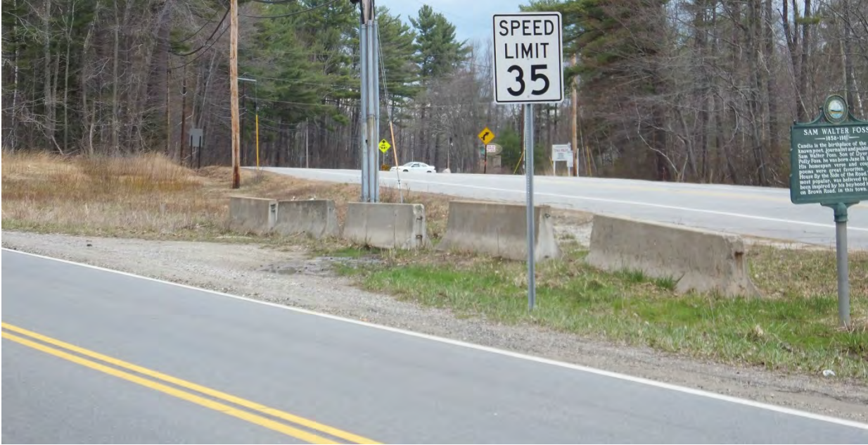
View of Main Street (left) and Raymond Road (right), looking north. Photo shows several roadside hazards including utility poles and concrete median barrier that is being used to discourage drivers from using the grass area as an unofficial intersection.
