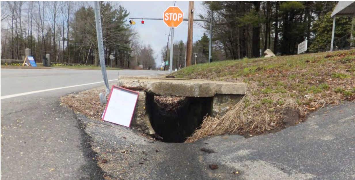
View of northbound approach on Main Street. Photo shows one of the two exposed drainage structures along the east side of the intersection.
