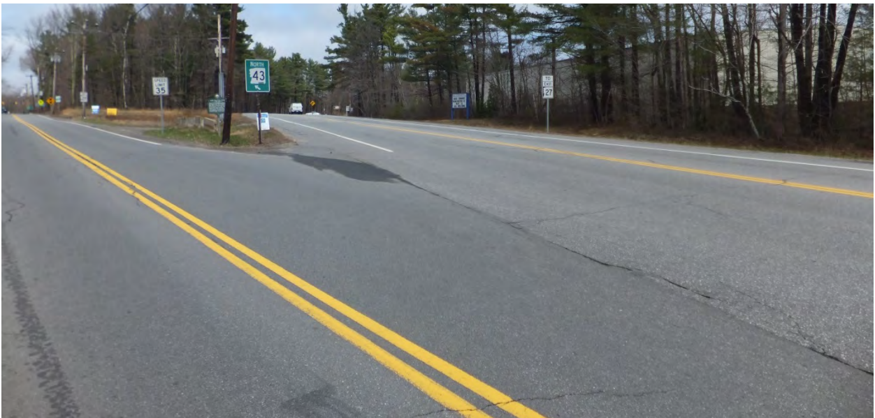
View from southbound Main Street approach looking north toward Raymond Road. The photo shows the severe skew of the intersection. Photo also shows the limited sight distance created by the crest curve.
