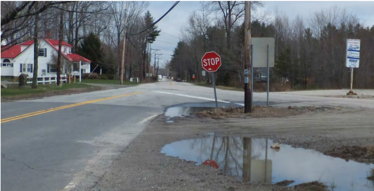
View of High Street looking east toward NH 27. Photo shows standing water on and along the intersection approach several hours after a rain event.
