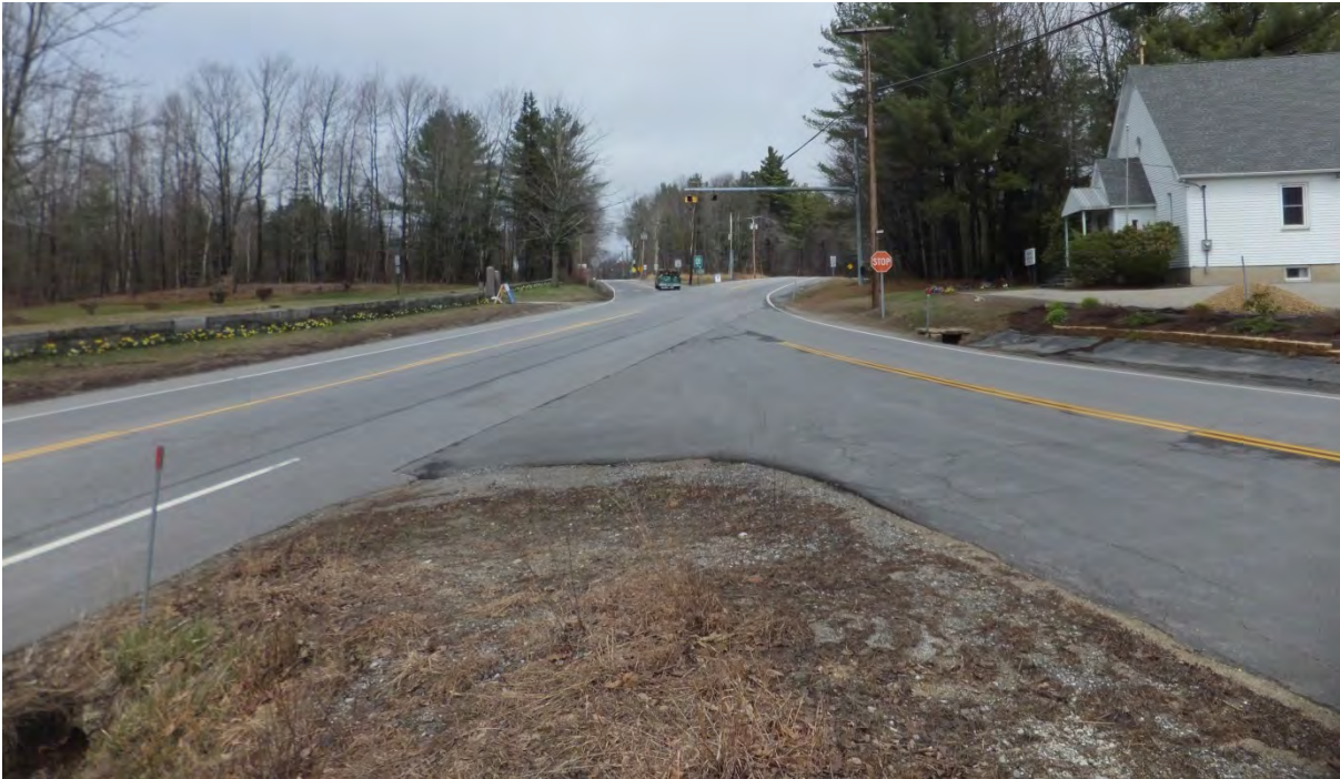
View of the intersection looking north from Main Street. Photo shows the discontinued edgeline from eastbound NH 43 onto southbound Main Street.
