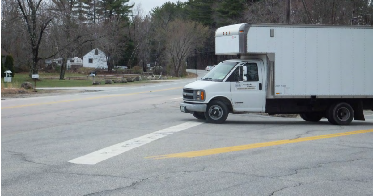
View of the intersection looking southwest from High Street. Photo shows the extended length of the stop bar and alignment of the centerline.
